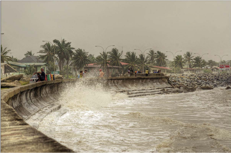
Figure 4. Seawall in Georgetown, Guyana. Photo: Richards, A. 2014. "Waves at Ogle." Accessed 10 June 2014. https://www.flickr.com/x/t/0092009/photos/arichards-gallery/6848905956/ . Creative Commons, Attribution-Non Commercial-NoDerivs 2.0. https://creativecommons.org/licenses/by-nc-nd/2.0/ .
